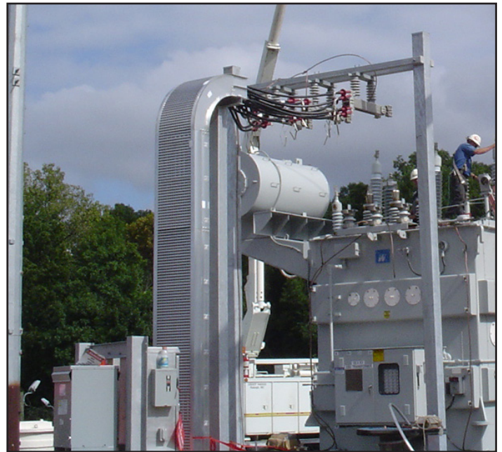
MP Husky 4000Amp, 5kV Cable Bus System with open air termination to GSU transformer.
